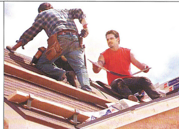
Terry McEwen, left, and Jim McEwen put standard 3-tab, asphalt shingles on the roof of the House Chronicles home in Van Buren Township.
